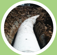
Concrete Pipeline for Drainage
